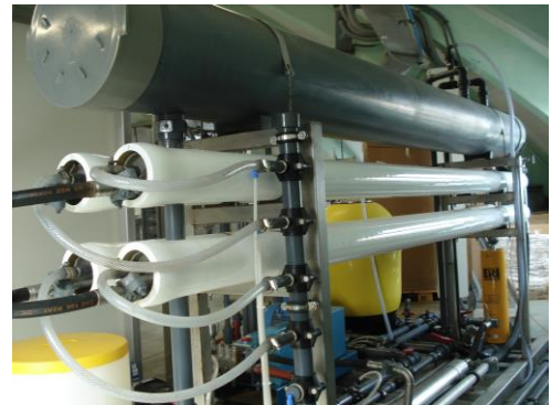
30 mcd solar PV powered RO plant
