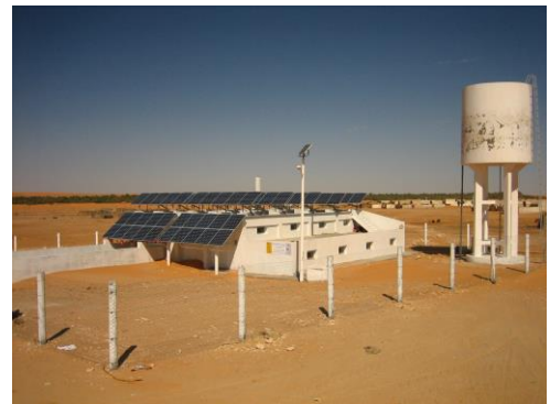
Autonomous solar PV-RO system installed in Tunisia
